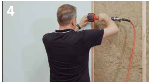
4 FIT LEFT TO RIGHT FROM A CORNER, OR FROM RIGHT SIDE OF A DOOR OPENING.
