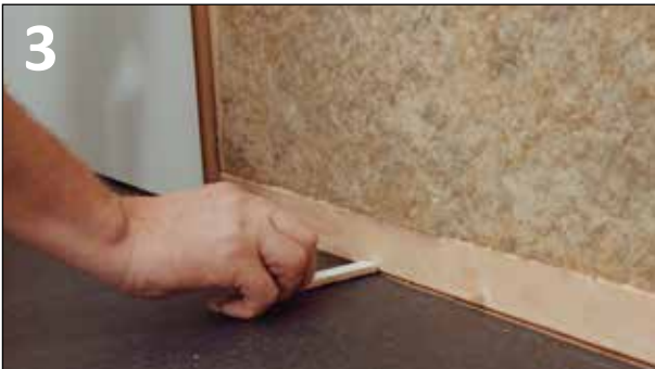
3 LIFT BOARDS 5MM TO 10MM UP FROM FLOOR.
